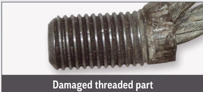
Loosening of external layer
